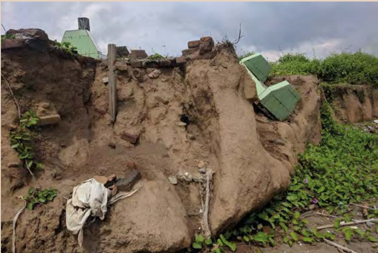
The damaged cemetery along the Takalar coast due to increased coastal erosion after the dredging by Boskalis. Photo credit: Both ENDS, 2019.
